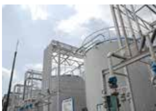
Varnish, solvent tank (Kyushu)
