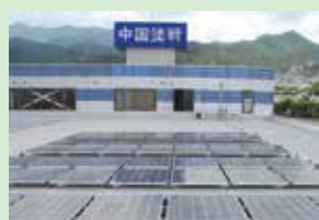
Solar Power Generation System (Headquarters in Hiroshima)
