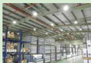
Changeover of lighting to LEDs (Kyushu Factory)
