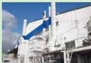
Ventilation equipment (Shiga factory)
