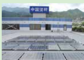
Solar Power Generation System (Headquarters in Hiroshima)
