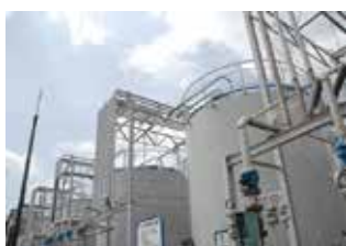
Varnish, solvent tank (Kyushu)
