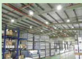
Changeover of lighting to LEDs (Kyushu Factory)
