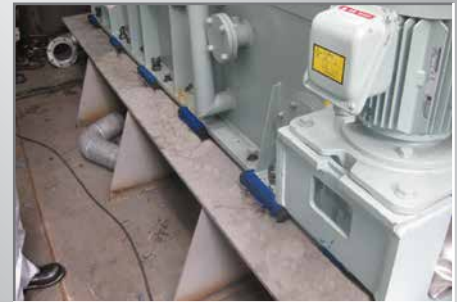
Under auxiliary machines, Generators
