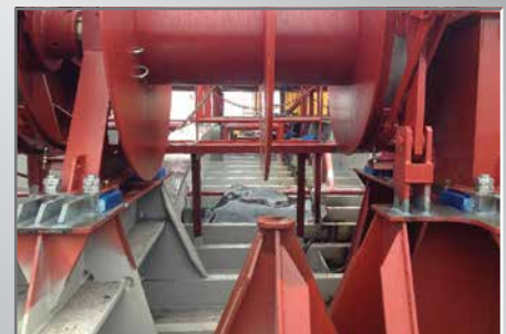
Under deck machines
